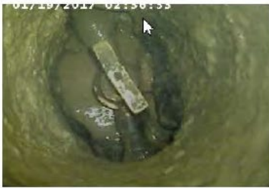
Lead Service Line
