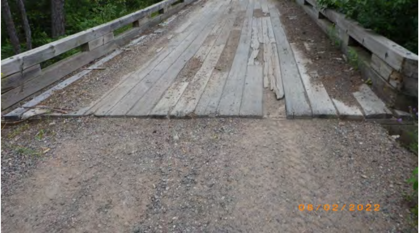
B2- West approach 2 inch settlement and CS3 deck boards.
