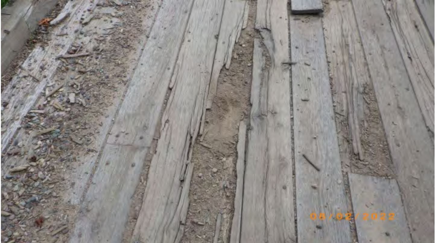
B1- CS3 rot and decay.
