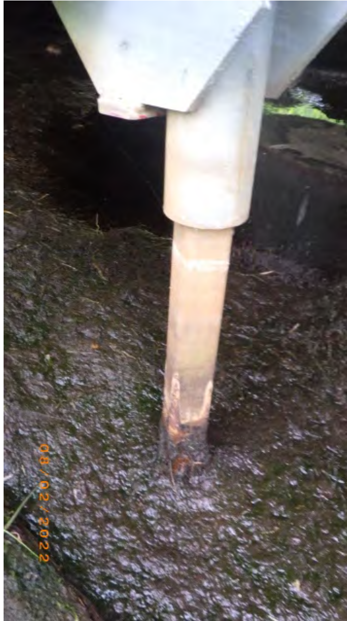
B1, Typical Helical, corrosion.
