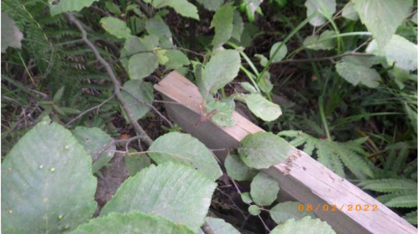
B4 Wingwall damage.
