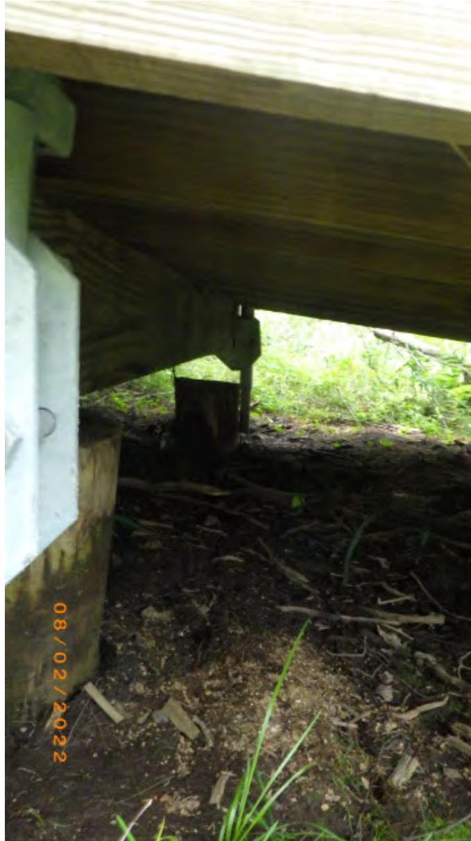
Bridge 2, East pier 15 degree lean.
