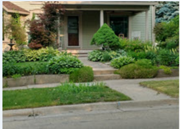
New Glarus used directional drilling to replace LSLs without disturbing homeowners’ yards. Photo credit: New Glarus Waterworks
