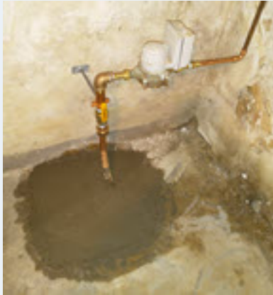
Basement in New Glarus after completing LSL replacement. Photo credit: New Glarus Waterworks
