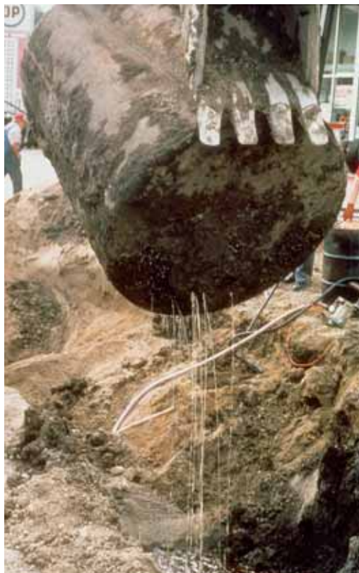
An aggressive program aims to locate, replace or remove buried tanks that can leak stored fuels. Few tanks leak this badly, but even small amounts of gasoline make water unfit for use in residences, businesses and for animals. Cleanups are expensive.
