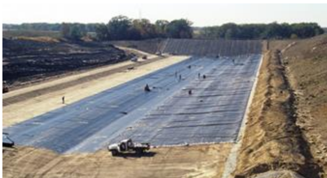
Installation of a compacted clay and geotextile liner at a landfill site in Wisconsin.
