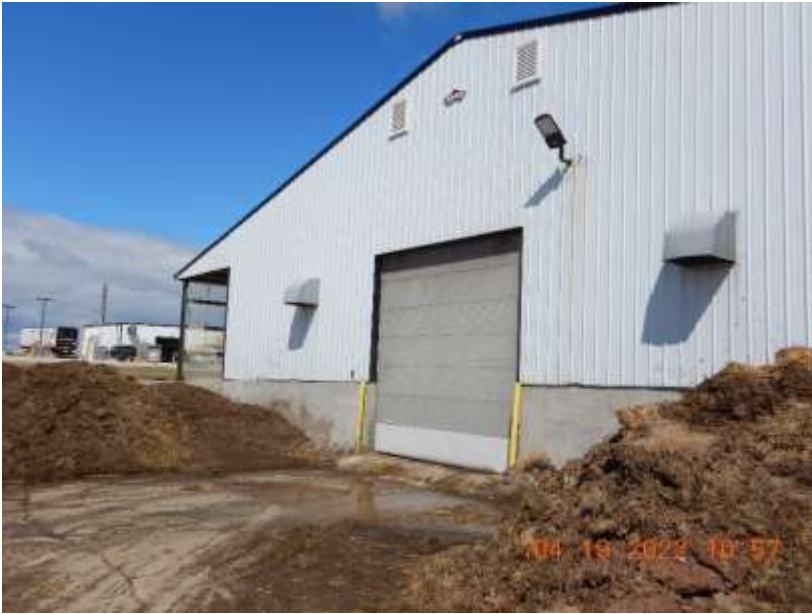
Photo 52. The shed where machinery is washed. Runoff from this area flows into the sand lane where it is comingled with manure.
